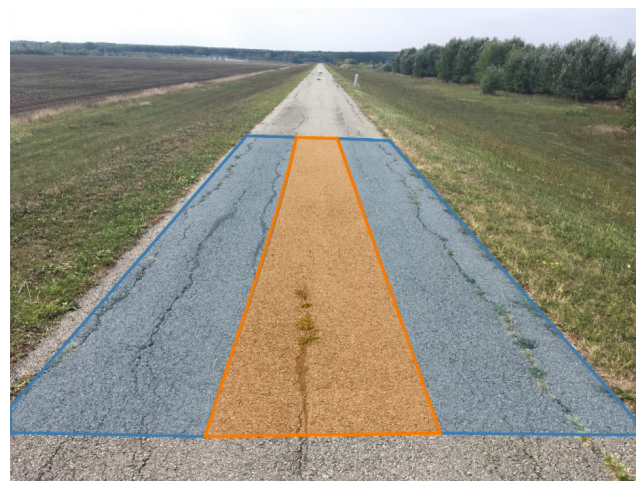
Figure 1 | Position of fissures on the paved dam crest Source: Nagy, 2019
