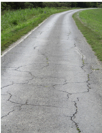
iii) Parallel + Perpendicular block cracks (b) Tisza, Left bank 55+300
