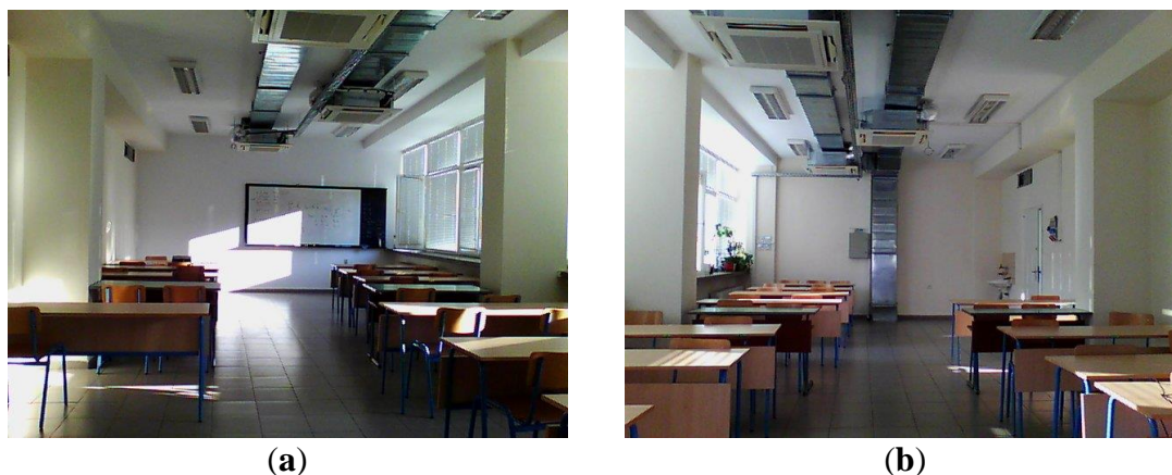
Figure 1. The university classroom with an HVAC system: (a) View to the front zone; (b) view to the back zone
