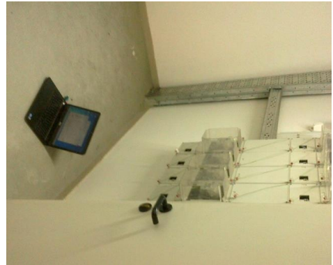
Figure 4. Receiver in electric meter room
