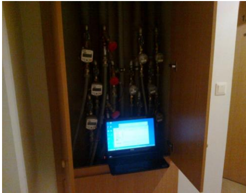
Figure 3. Receiver in water and heating meter cabinet
