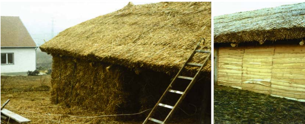
Figure 14-16 Placement of fodder insulation in a cost-effective cow shed in Bercel (architect: Dr. Gábor Ónodi)
