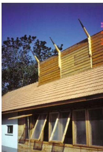
Figure 30 Convertible foiled framed windows of simple pig sheds in Kenderes with natural ventilation, lighting and heat protection and heat preservation (architect: Dr. Gábor Reischl)
