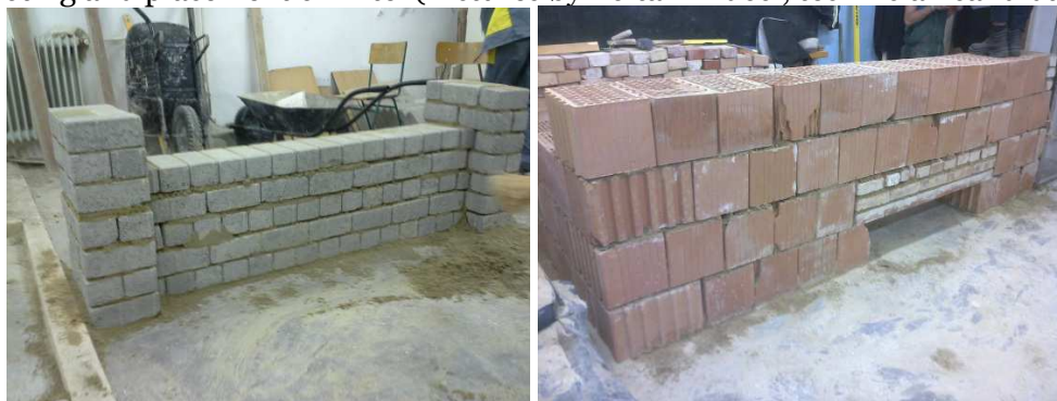
Figure 1. Student workroom products. Completed sub-tasks: construction of fence footing and placement of lintel (Pictures by Zoltan Erdósi, technician candidate)
